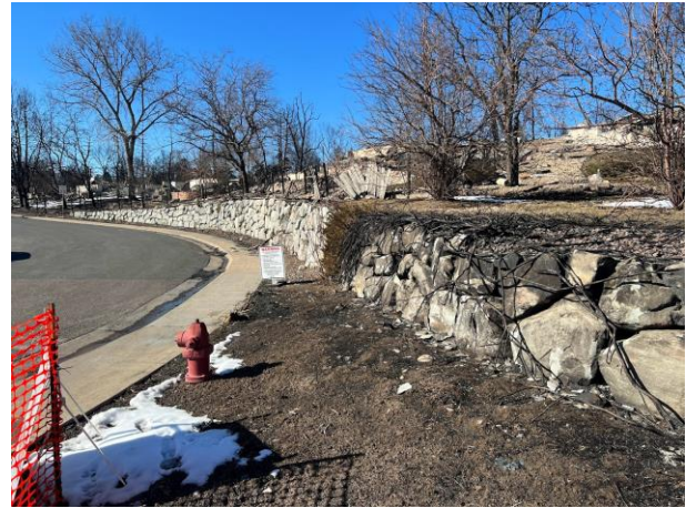
(b) Displaced blocks at Via Appia and Eldorado Ln (39°58'27.8" N, 105°09'41.9" W)
