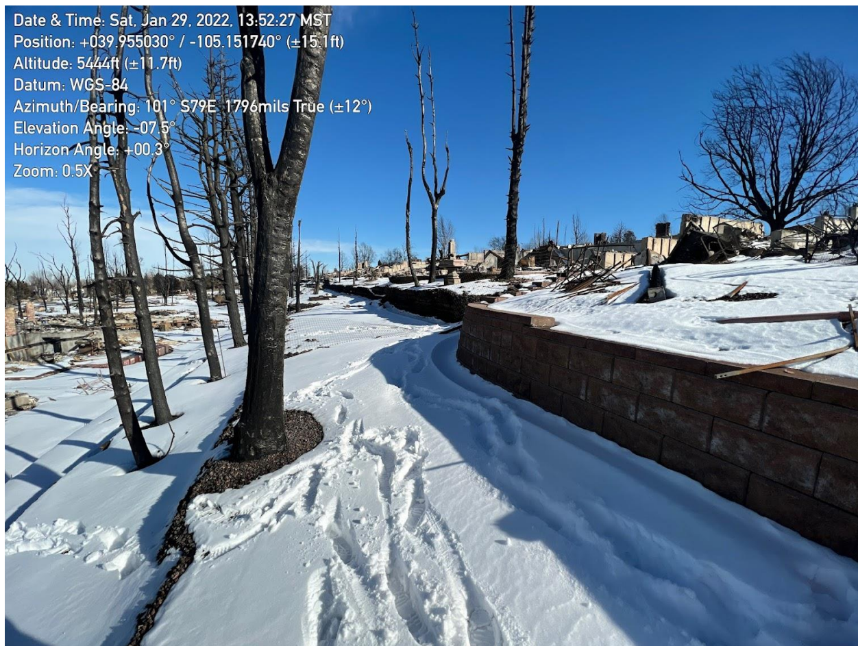
Figure 6-13. Backyard retaining walls behind houses along the north side of St. Andrews Ln showing good performance of masonry block wall (foreground) relative to fully burned tiers in the background and below (39°57'18.1" N, 105°09'06.3" W)
