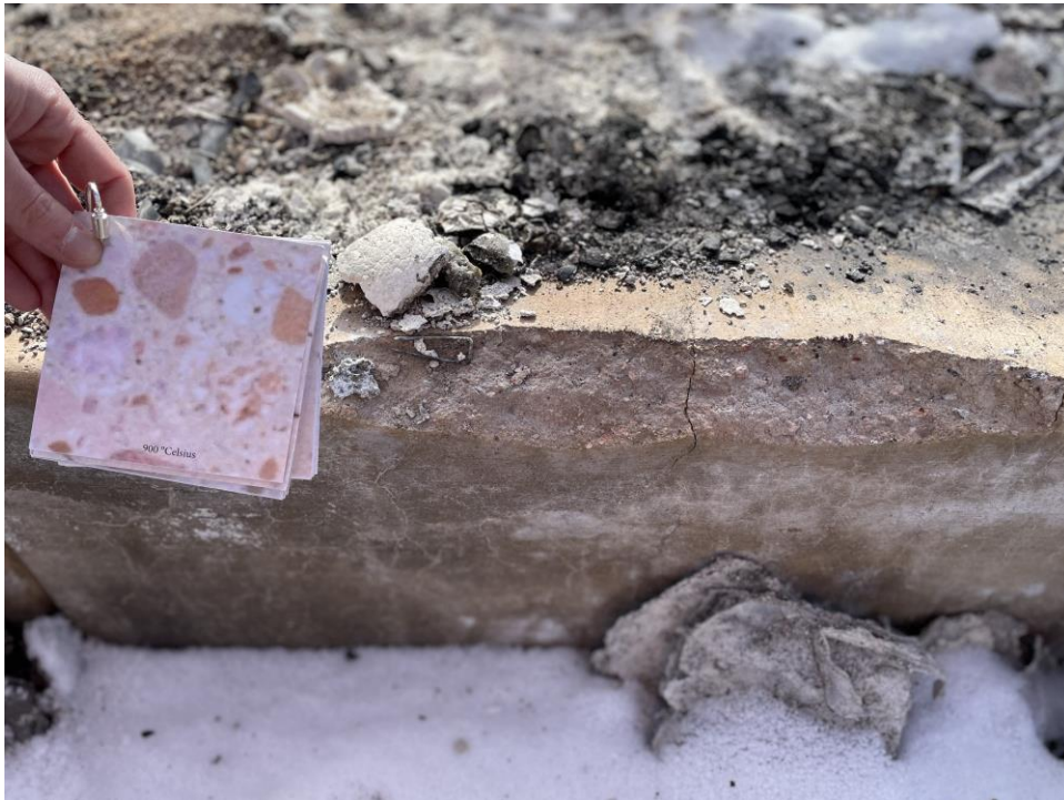
Figure 2-6. Comparing concrete colors from Hager (2014) to foundation colors in the field (39°58'20.0" N, 105°09'22.2" W)
