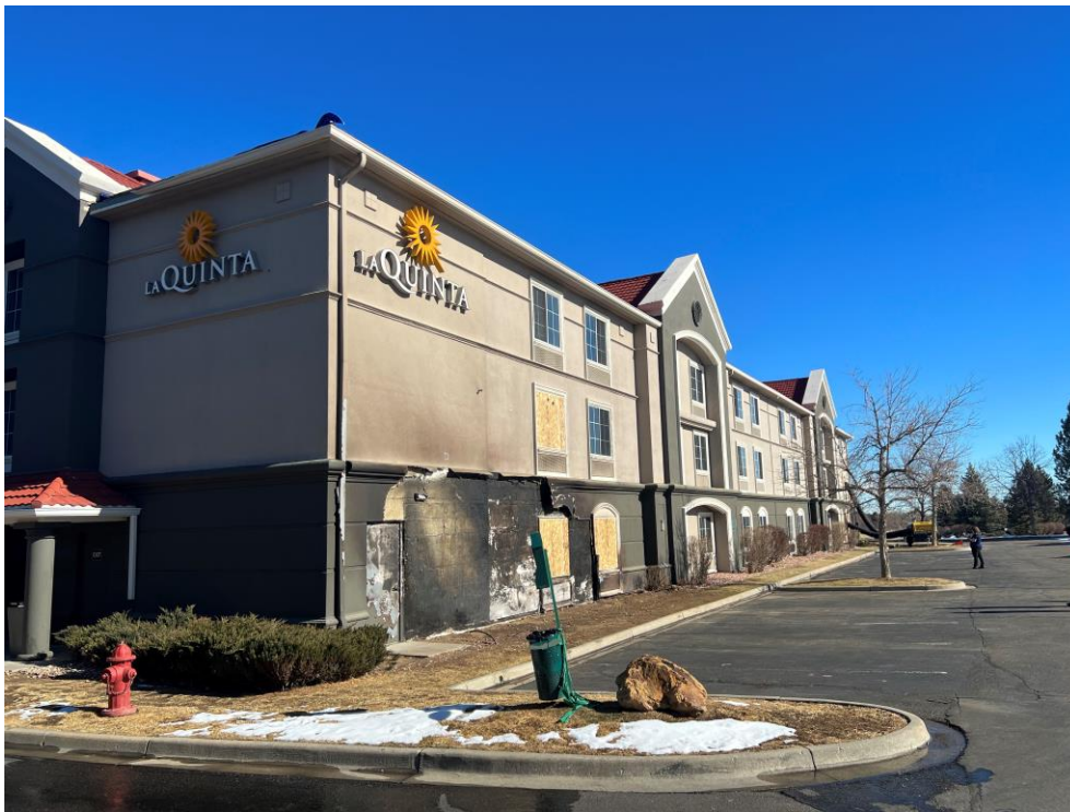
Figure 8-28. Damaged La Quinta Inn in Louisville, along Highway 36 (39°57'32.2" N, 105°09'43.6" W)
