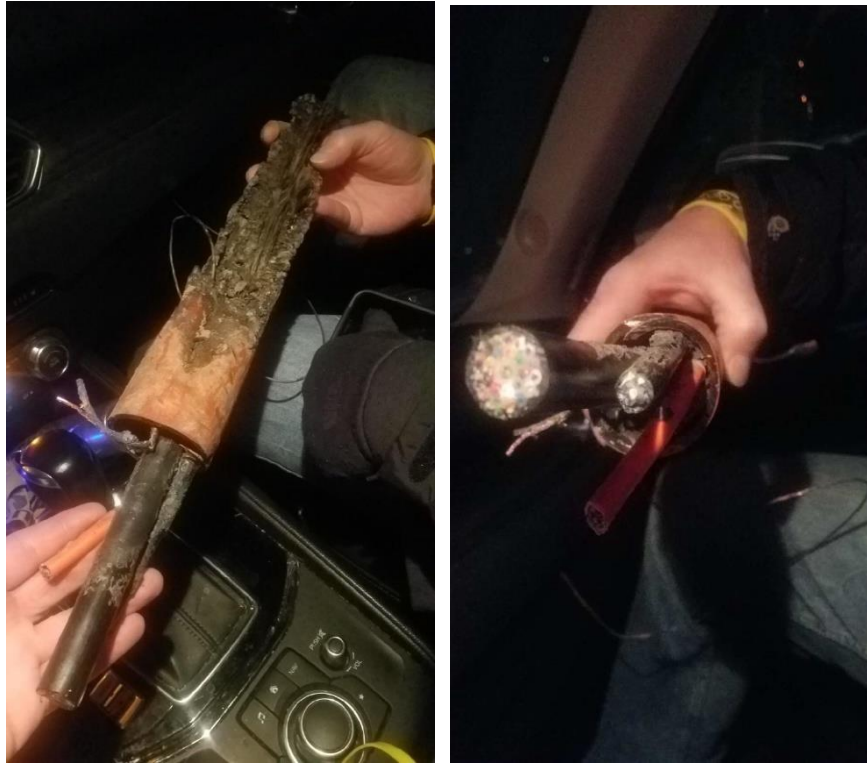
Figure 7–3. Damaged fiber optic cable linking Louisville water treatment plants (approximate location: 39°58'30.6"N 105°09'57.7"W)
