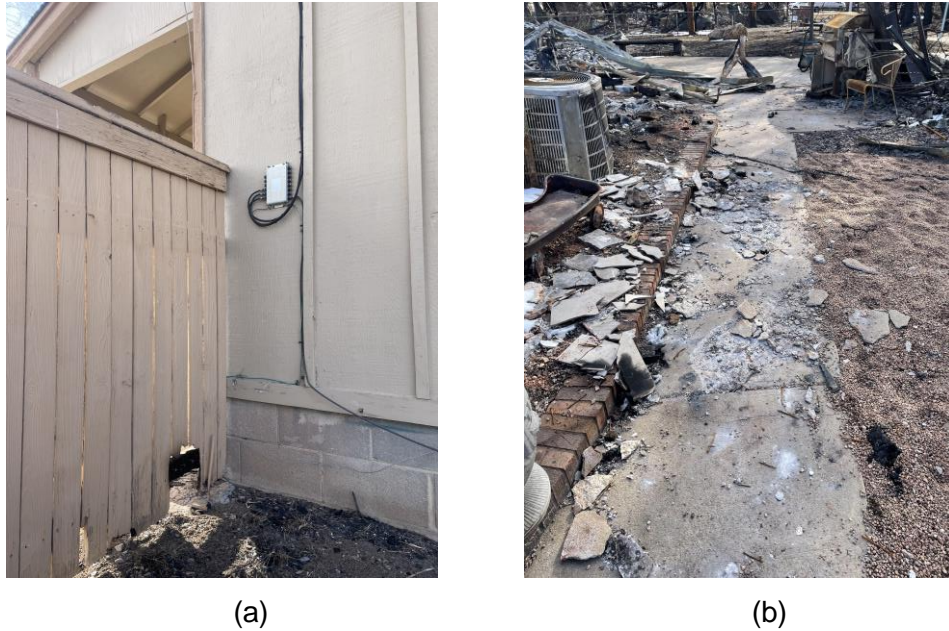
Figure 8-21. Housing characteristics in Original Town Superior (a) burnt fences touching homes and (b) spalling of concrete sidewalks (37°57'12.204" N, 105°10'4.368" W)
