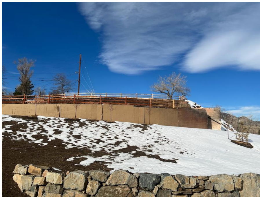
Figure 6-15. Reinforced concrete wall at corner of Marshall Rd and Eldorado Springs Dr. (39°57'22.3" N, 105°13'46.4" W)
