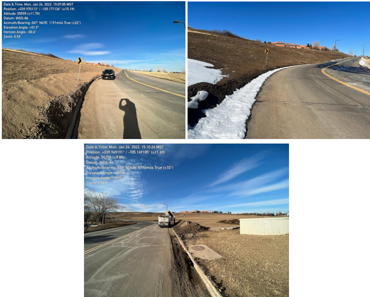
Figure 6-17. Images of soil erosion along Century Blvd. (39°58'12.4" N, 105°10'16.1" W)
