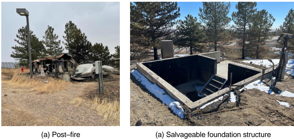
Figure 7-5. Destroyed backup generator at Superior Water Treatment Plant (39°56'33.8" N, 105°09'50.2" W)
